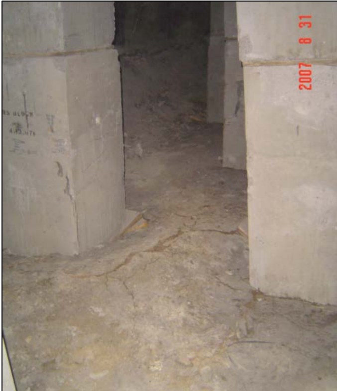
Figure 7. Excessive floor heave and cracks on the floor.
