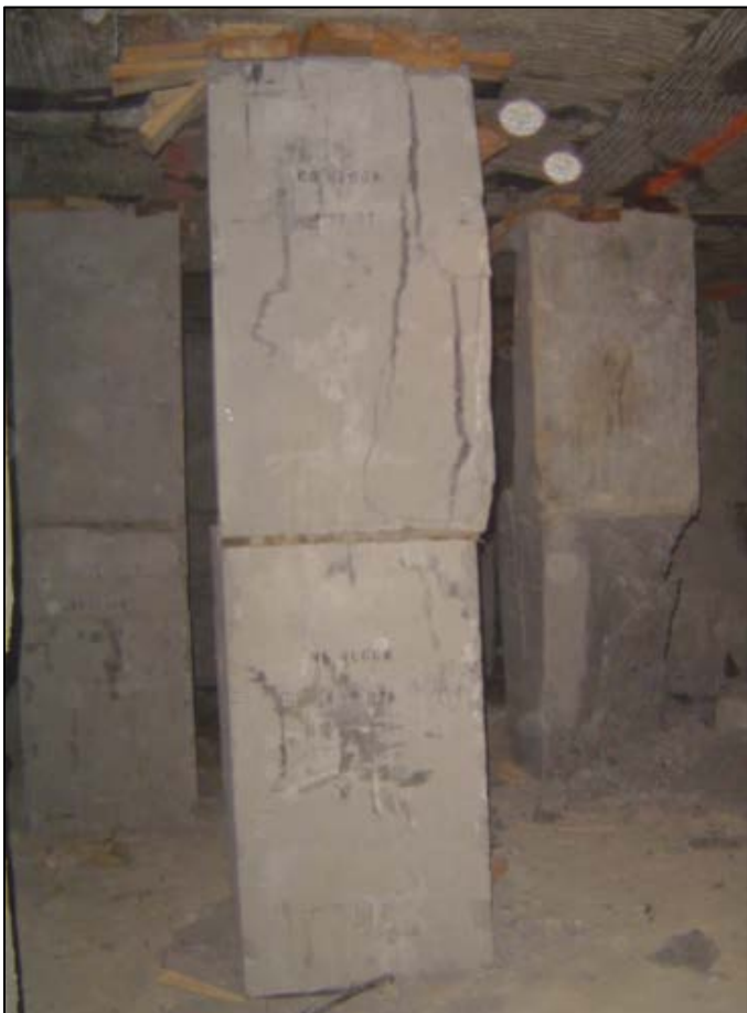
Figure 8. Failed crib at the Recovery Face.
